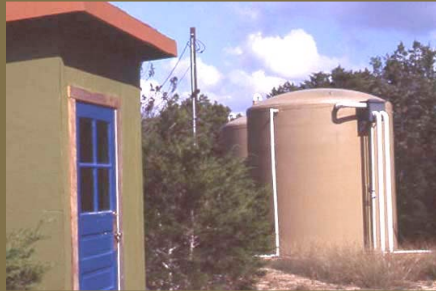
2 10K gallon rainwater collection system
